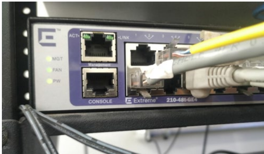
Figura A 3. - SWITCH de red Extreme Network.
